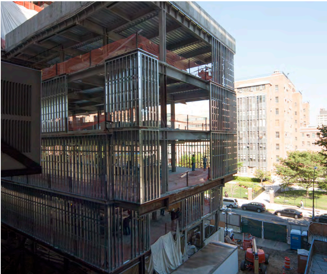
Downstate’s new Public Health Academic Building under construction. It will open in 2016.
